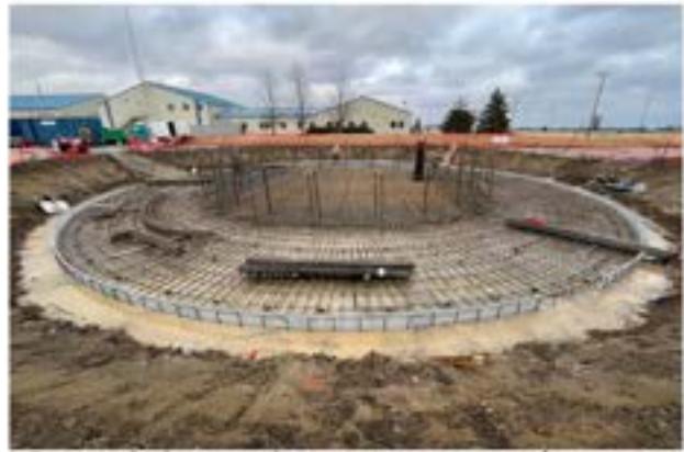
Pictured above is the construction site for a new 2-million-gallon elevated tank, which will serve a new data center being built next to The District's property in Wood County..
